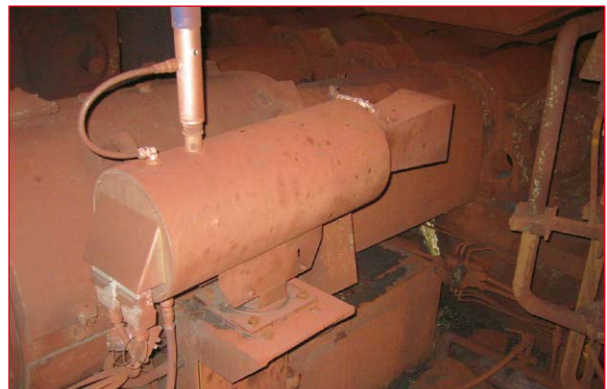
Infrared acquisition unit
